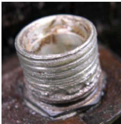
Poor thread condition of the old condenser fitting suggests it is cut on fitting and explains the significant effort required to tighten the joint.
