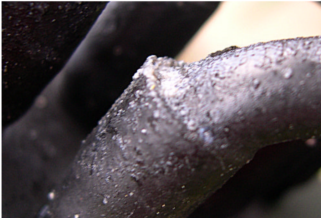
Badly corroded joints in the condenser matrix pipework are a like source of a gas leak.
